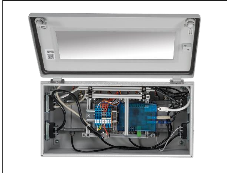
Figure 11: Control cabinet open
